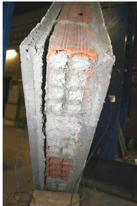
b) Detail of the detachment between the strengthening overlay and the substrate observed in specimen armo_02
