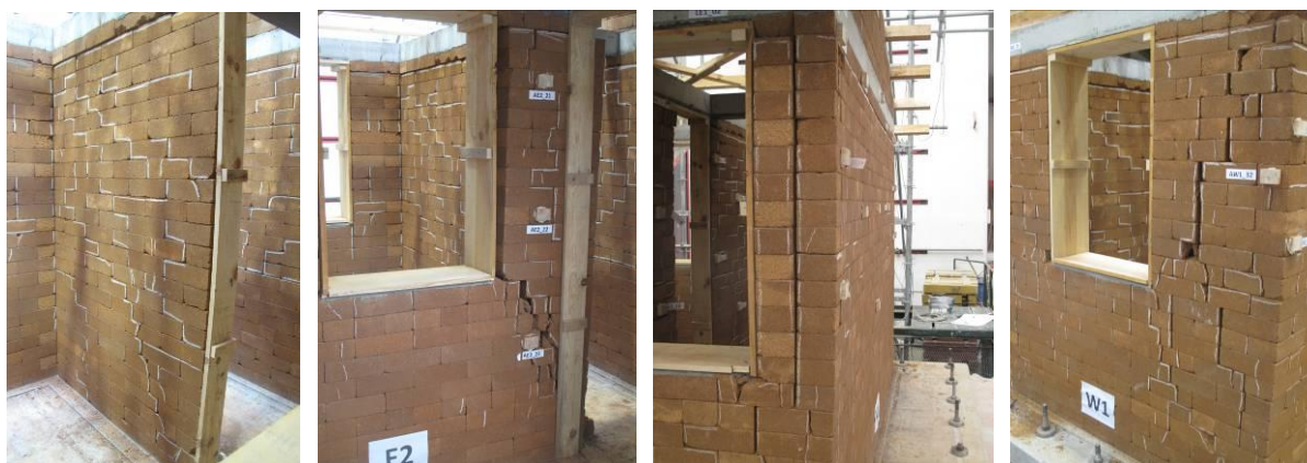
Figure 6. Crack pattern: a) inner wall, b) East pier, c) South-East and d) South-West corners
