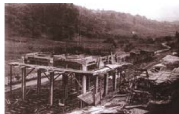
Figure 5 - Construction detail of coal silos in Alcanadas mine, 1941. Unknown author; coll. Victor Guerra
