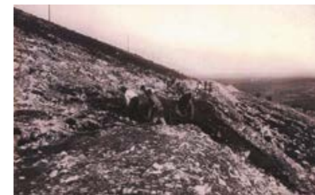
Figure 4 - Preparatory work for the railway platform, in the hills of Pevide (Porto de Mós). AHGM, LNEG
