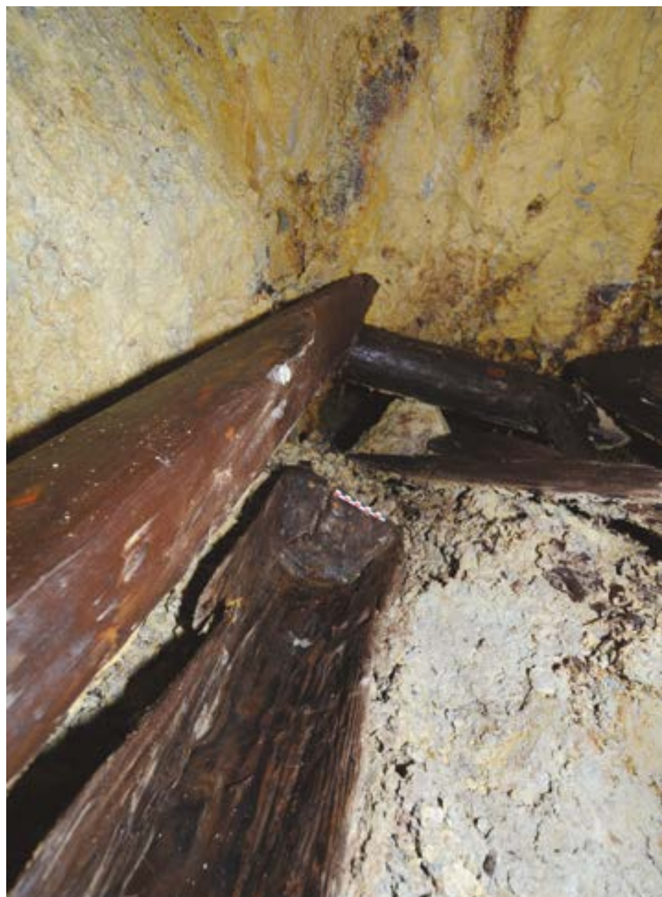
Figure 9 The wooden channel that collected the water from the upper water wheel in Catalina Monulesti mine still at its place along the wheel (Photo. C. Tamas).
