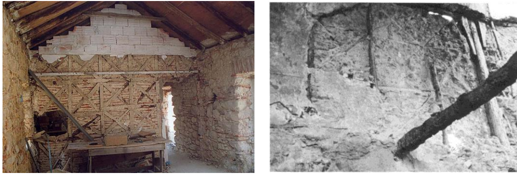
Figure 4. (left) 'Pombalino' wall in a house in Alcácer do Sal, Portugal [12]; (right) Internal wall showing the timber frame structure characteristic of the 'casa baraccata' system in Calabria, Italy [16]
