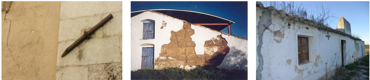
Figure 8. (8a-left) Metal ties can be easily found all over Italy [17]; (8b-middle) Tie-rods on a gable rammed earth wall in Safara, Portugal [12]; (8c-right) Tie-rods in vernacular building in Melides, Portugal (Photo by CI-ESG, 2013)
