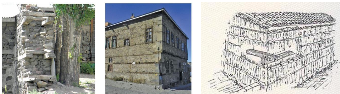
Figure 5. (5a-left) Timber horizontal elements, known as ‘hatil’, embedded in a masonry wall in Turkey [19]; (5b-middle) Traditional house with horizontal timber beams in Erzurum, Turkey [19]; (5c-right) Horizontal timber elements embedded in rammed earth wall in Alentejo, Portugal [23]
