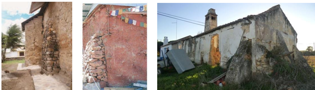
Figure 9. (9a-left) Stone buttress in adobe masonry chapel in Peru [28]; (9b-middle) Rubble stone corner buttress reinforcing the earthen walls of an ancient Buddhist temple in the Western Himalayas in India [29]; (9c-right) Buttress reinforcing a ruined rammed earth vernacular construction in Melides, Portugal (Photo by CI-ESG, 2013)
