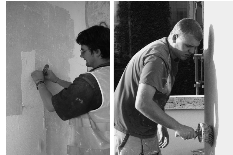
FIG. 18 Upper terrace, north-east facade, pilot work in 2011; Michal Pech removes the ammonium-compresses, which served to remove the gypsum crust. Photo Ivo Hammer 2011.
