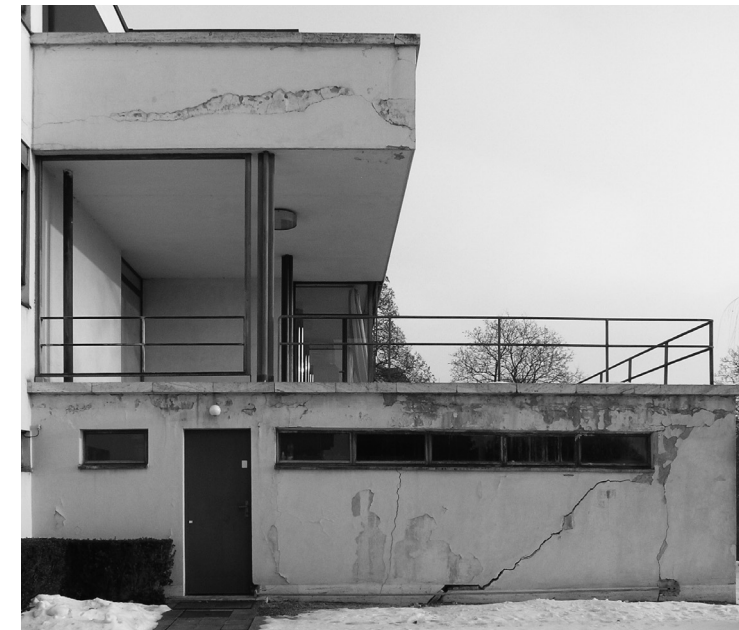
FIG. 17 Northwest facade, detail. Static defects of the lower terrace, caused by a leaky drain pipe. Damage to plaster and painting from 1985 by deficiencies in the drainage, harmful salts and a paint material that is not compatible with the previous lime washes. The former lime washes are partially dark by dirt and by environmental conversion of the lime into gypsum. Photo by Ivo Hammer, 2005.
