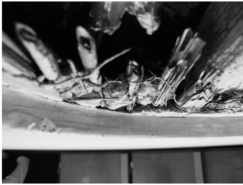
FIG. 14 Fritz Tugendhat bedroom. Opening in the ceiling, where light fixture has been removed. The prefabricated cane mat is suspended from the concrete floor structure above and supported by a wire mesh. Photo by Ivo Hammer.
