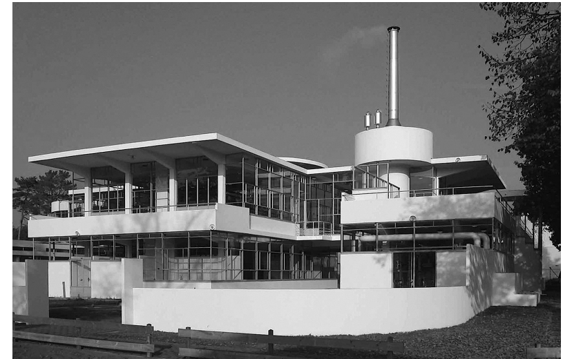
FIG. 11 Zonnestraal sanatorium brought back to life became the icon of a successful approach to conservation based on sensible reuse, historical documentation and technological expertise. Photo by Benedetto Di Cristina
