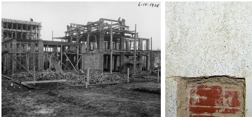
FIG. 5 Fairgrounds, Pavilion of Arts and Crafts School in Brno by Pavel Janák during construction (1927– 28). Brick-clad concrete base, hollow block brick wall, wood chip board, steel girders.
