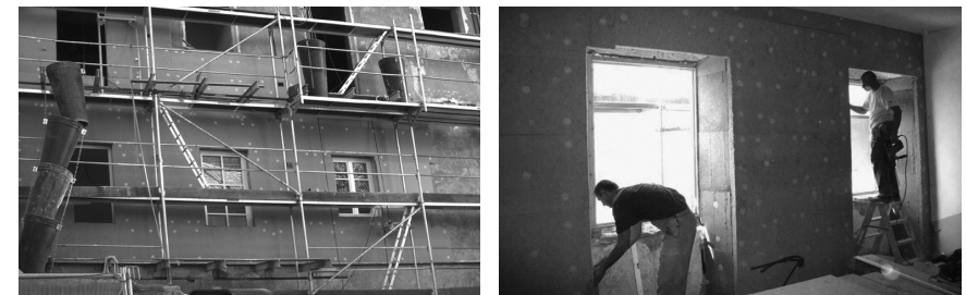
FIG. 7 External thermal insulation composite system (ETICS). Photo by Arch. Dietmar Dejori.
