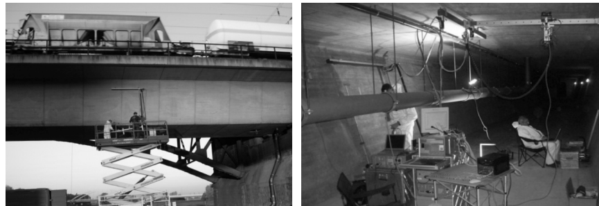
FIG.4 Applying advanced non-destructive methods to a German railway bridge. Use of GPR, ultrasonic and impact-echo techniques in the same area to obtain a geometrical accurate correlation.
