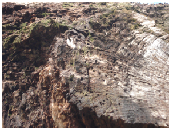
Figure 5. Detail of the degradation stage of the left edged of the beam.
