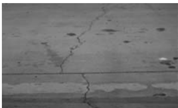
Figure 20. Transversal crack in cement concrete pavement (Source: Fig. 8, Teltayev 2013).
