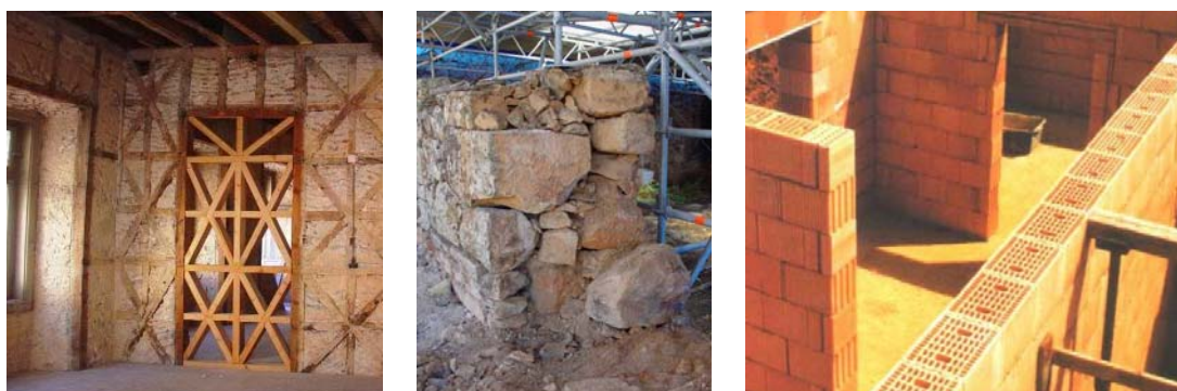
Figure 1. Examples of different masonry types (from left to right): timber braced “Pombalino” system after the 1755 earthquake in Lisbon; irregular stone wall with a complex transverse cross section; unreinforced masonry using blocks complying with thermal and sound regulations.
