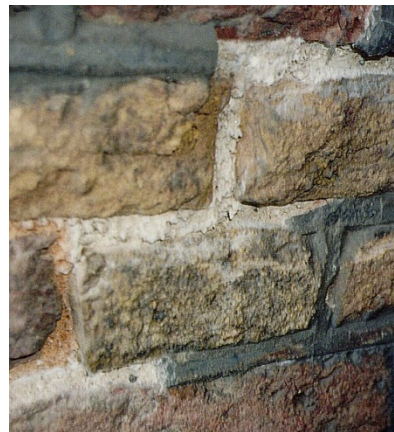
Fig. 6 Push-out of cement re-pointing due to crystallization of salts at the interface of new pointing and old bedding mortar.
