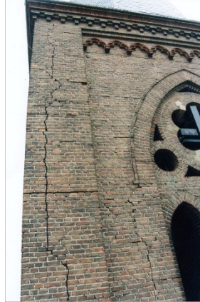
Fig. 11: Damage pattern that may at easily attributed to a structural mechanism.
