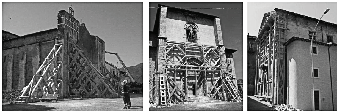
Figure 6. Examples of different temporary solutions applied according to the local situation (Modena et al. , 2010).
