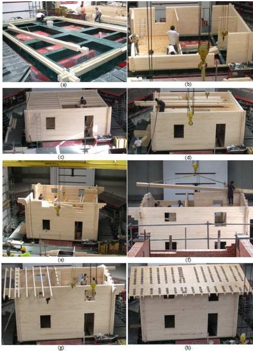
Figure 3 Stages of construction (a) connecting the bottom logs with the steel lattice (b) laying the ground floor walls (c) placing interstorey floor beams (d) nailing OSB planks to the floor joists (e) laying the first floor walls (f) positioning the ridge board (g) connecting the roof rafters (h) Completed house
