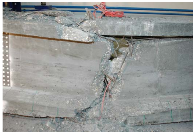
Figure 9: Failure mode observed in girder STR_PRE.
