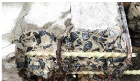
a) GFRP bars after 12 months
