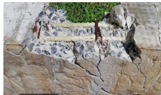
b) GFRP bars after 60 months
