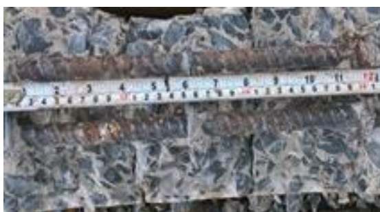
c) Steel bar after 12 months
