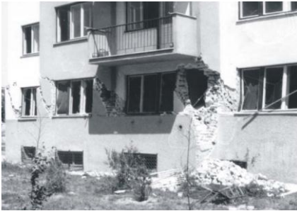
Figure 10. Concentrated damage at the ground floor (Petrovski, 2003).
