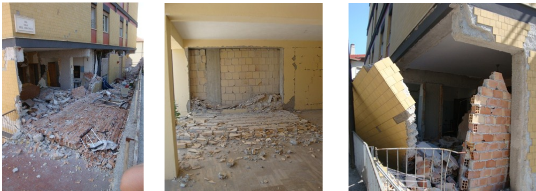
Figure 2. Failure patterns of masonry infill walls found in the recent earthquake of L'Áquila
