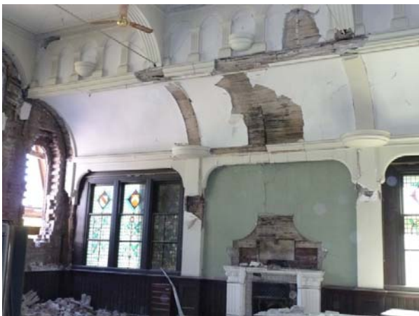
Figure 4: Damaged zone below the roof structure
