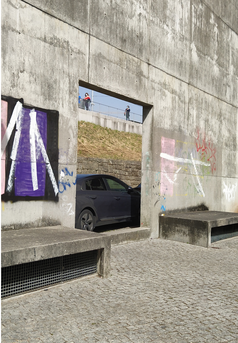
Figure 3.2.8. Photograph taken in Bouça neighbourhood. Passage through the concrete wall on the ground floor.
