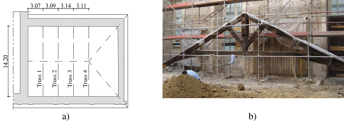
Figure 3: Wing 1 from Chimico laboratory: (a) plan with location of trusses; (b) photograph of truss #4 once it was moved down
