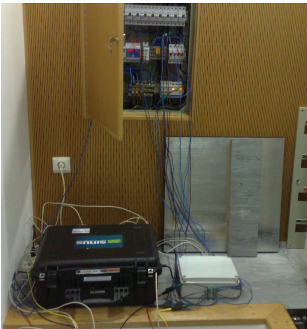
Fig. 2- Electric Power Quality Monitor installed next to an electrical switchboard.
