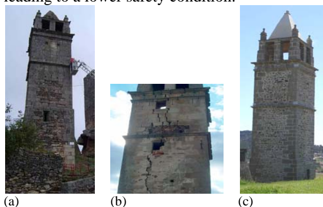
Figure 1 – Mogadouro Clock Tower: (a) and (b) general view of the tower with severe damage; and (c) the tower after the strengthening works
