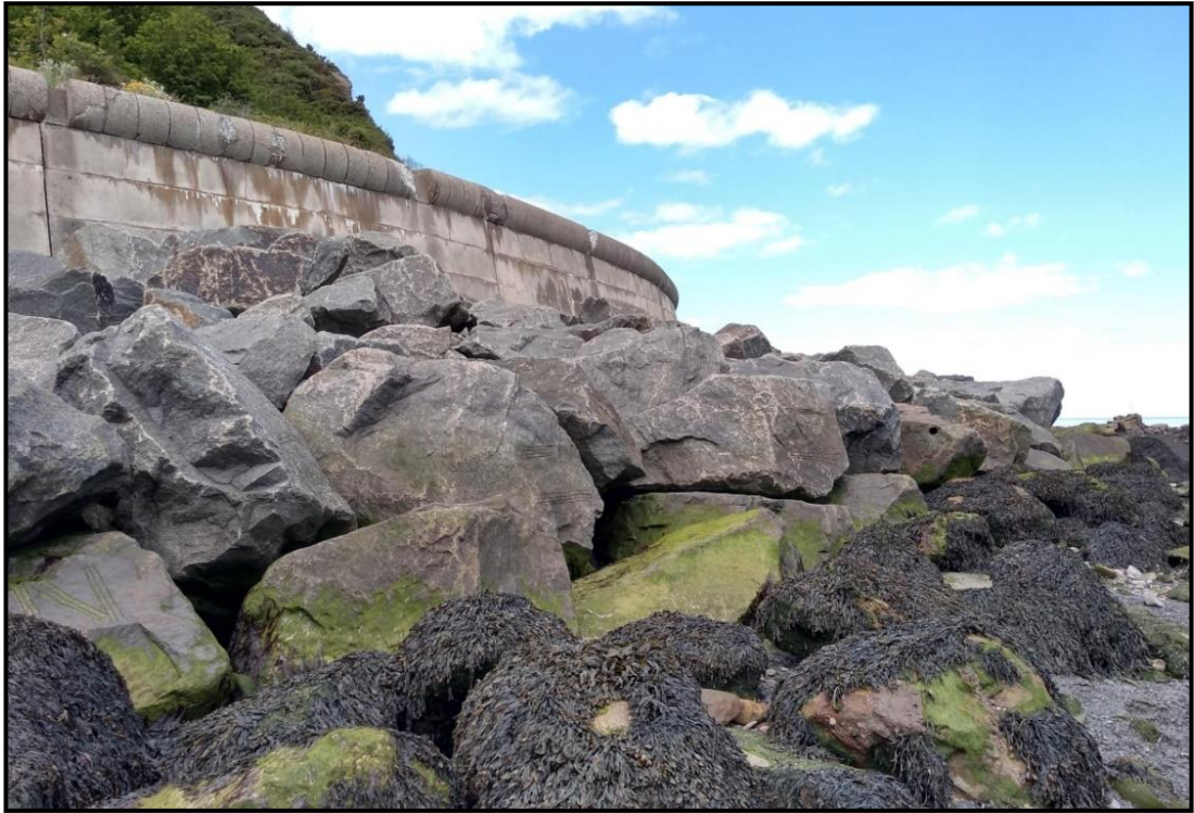
Figure 1.1 – Section of the rock armour created as part of the Runswick Bay Coastal Protection Scheme (taken at beginning of the study in February 2019).
