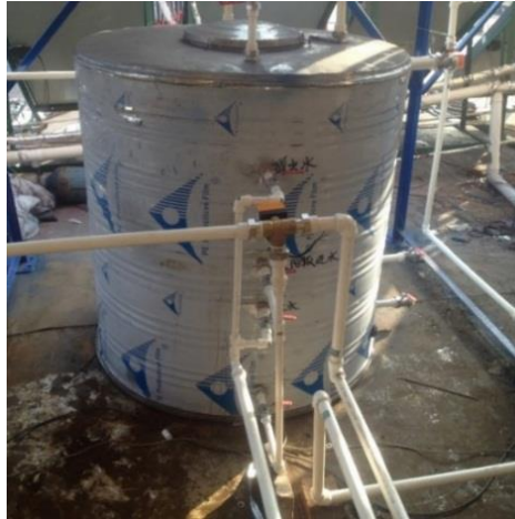
Fig. 5- 12 : Image of the heat tank
