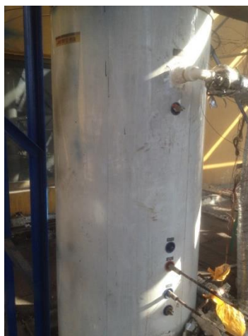
Fig. 4- 3: Image of the condenser
