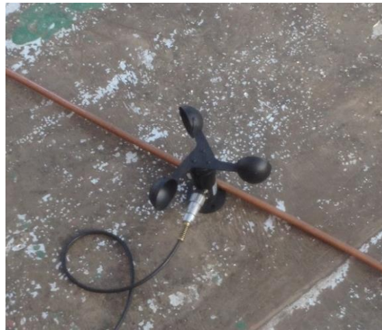
Fig. 4- 11: Image of the anemometer
