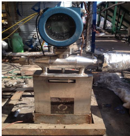
Fig. 4- 7: Image of the mass flowmeter
