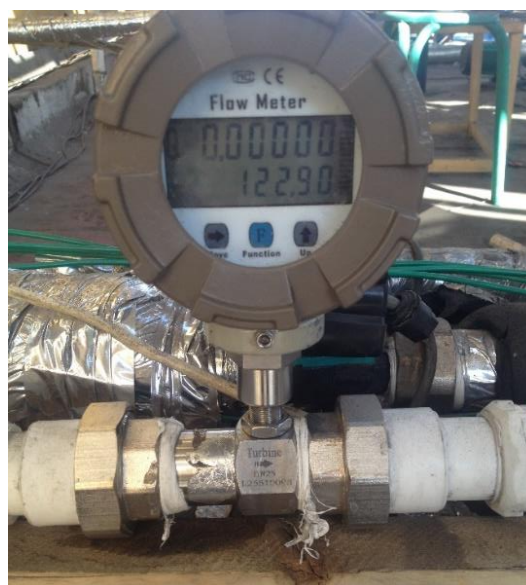
Fig. 4- 6: Image of the water flowmeter
