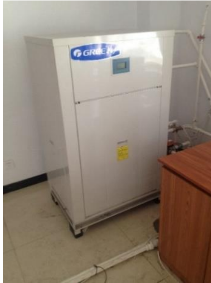
Fig. 5- 13: Image of the heat pump
