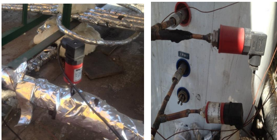
Fig. 4- 8: Image of the pressure transmitter
