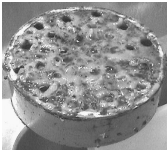
Figure 6. Liquid distributor showing the growth of biomass on the lower surface. On the top side, that occurrence was even stronger.
