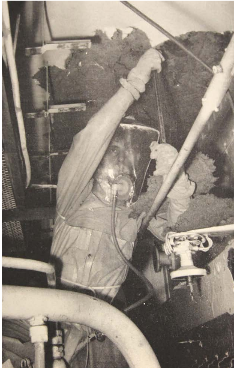
Figure 5.3 Removing lagging. Here we not only see the fibrous asbestos being removed, but also the cramped and obstructive conditions that work was undertaken in. This provides some context for workers resisting bulky protective equipment that made their jobs harder and made hot and claustrophobic conditions worse. Source: Working With Asbestos (black and white).
