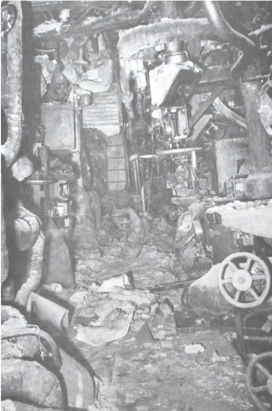
Figure 5.0: Removal of asbestos pipe lagging in a ship's boiler room (Devonport Dockyard). This photograph illustrates some of the comments made by former Dockyard workers about the level of dust and debris around them when asbestos was being removed. As well as the dust that we can see in this photograph, there would have been airborne dust particles, small enough to be inhaled by workers. It was used by Harries to highlight how dusty the removal of lagging was in support of his MD thesis.
