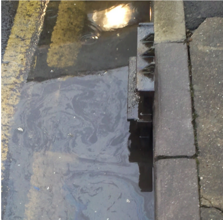
Figure 2.4 Blocked gully showing water backing up.
