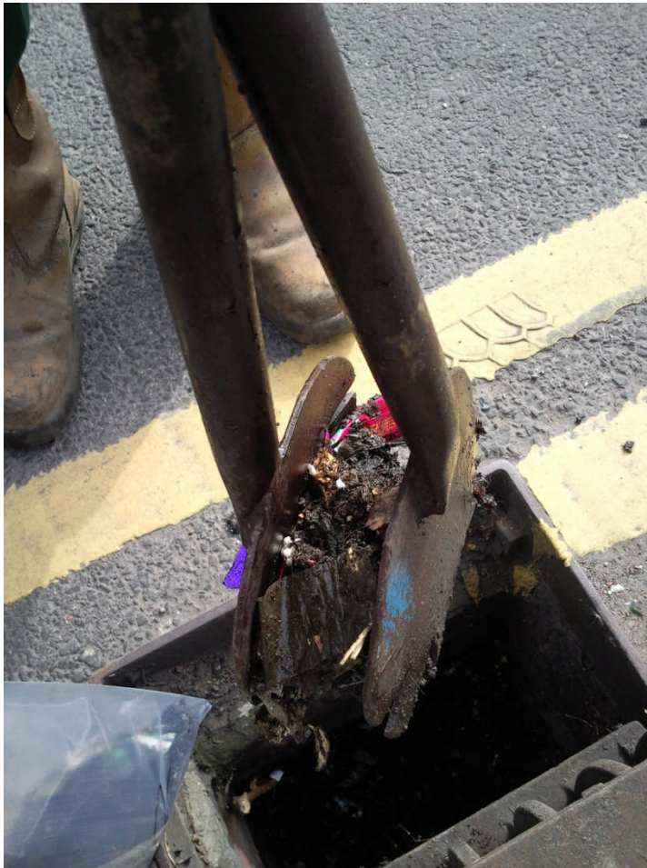
Figure 3.1 Sample from the gully pot being removed using the long gully grabs.
