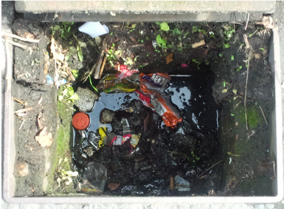
Figure 2.3 Large particle and rubbish littered within a gully pot.
