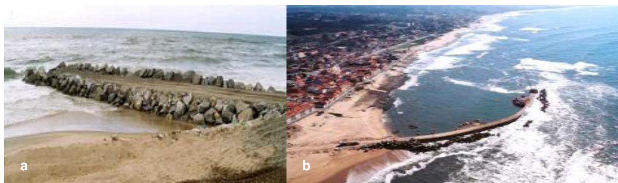
Fig. 2. Construction of the Aguda breakwater: a) access groin; b) final works (adapted from INAG, 2010)
