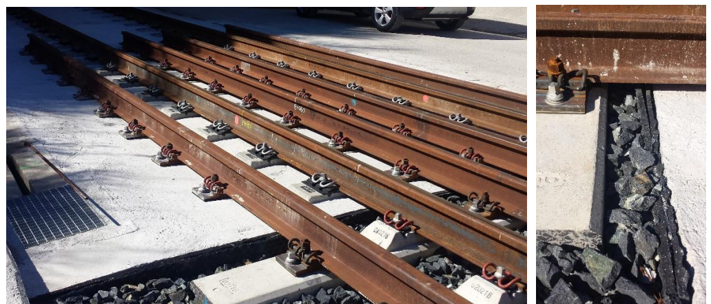
Figure 2. Detail of cross-section of the ballast mat between slab and ballast track in Dinatrans solution.
