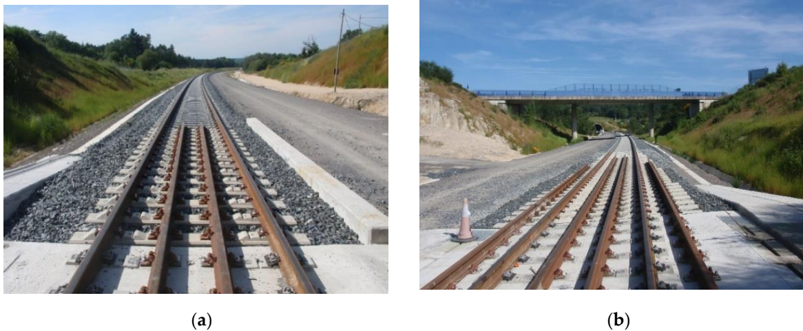
Figure 1. (a) Common solution for track transition used in Spain. (b) Dinatrans track transition.
