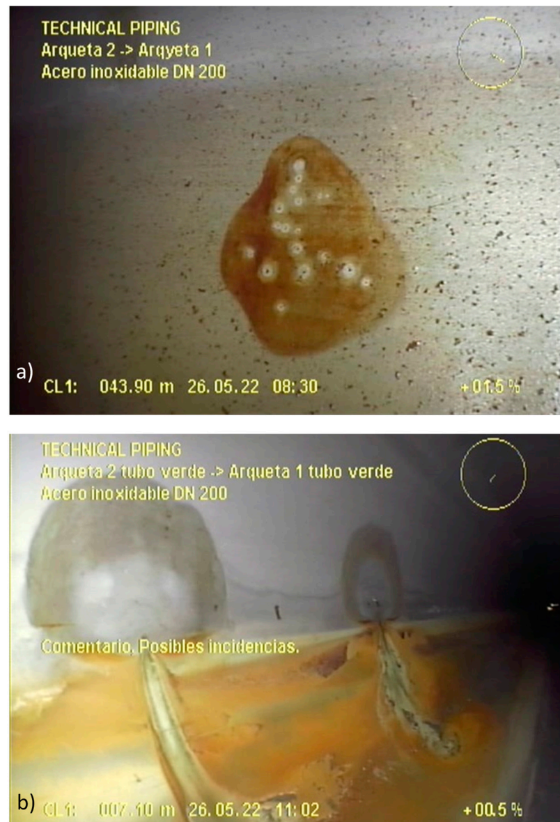
Figure 5. Video-inspection image of the interior of the piping system. (a) Detail of pitting; (b) detail of “mushroom-shaped” marks around two pits.
