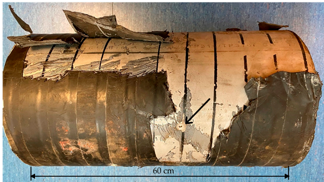
Figure 1. Sample of pipe extracted from the port piping system; a through-wall pitting can be observed in the center (black arrow).
