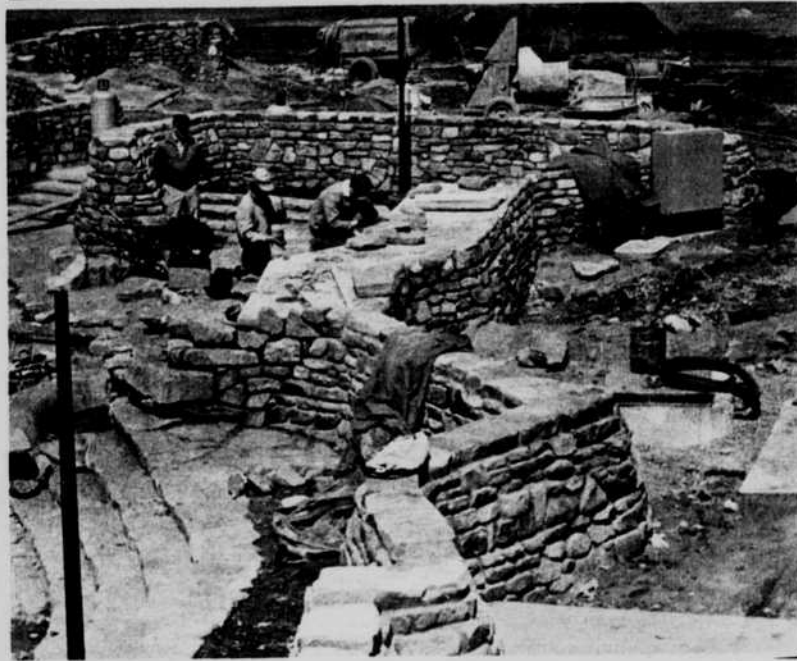
Stonework construction on the north side of Parkland's Campus continues and could be completed as early as the middle of next month. Photo by Mike Haberkorn.
