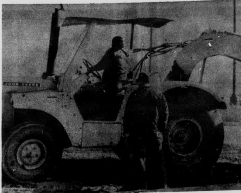
WORK ON CAMPUS continues as planned. All perimeter roads have already been completed, and grass seeding has started on the landscape surrounding the campus area. Indoor work is also proceeding well,
