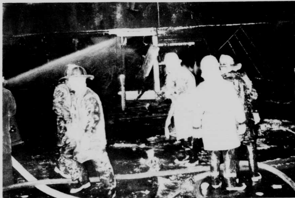
As soon as the fire is under control the anticlimatic and tedious job of cleanup begins.
