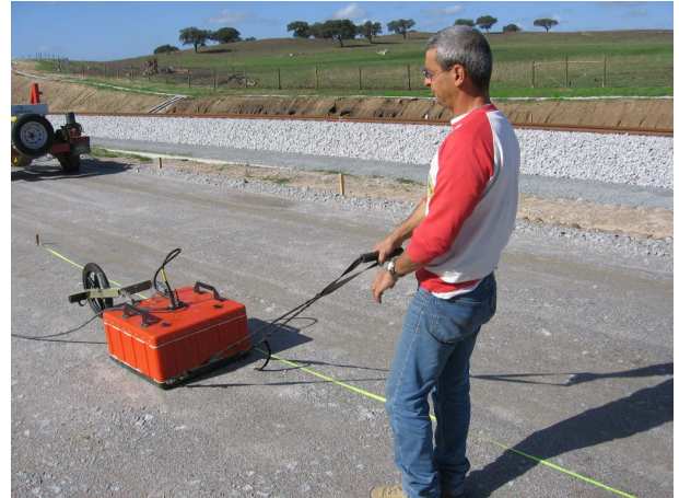
Figure 2 – Partial view of the trial embankment with execution of a GPR profile.
