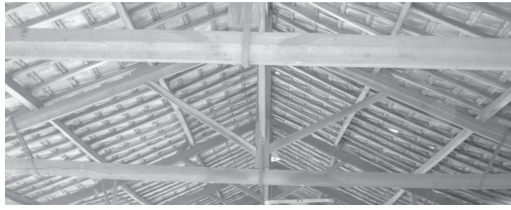
Figure 1. Incorrect truss configuration for the roof span.
