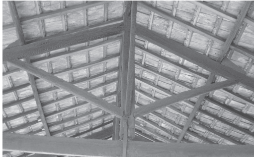
Figure 2. Wrong positioning of the purlins with eccentricity relatively to the truss joint.
