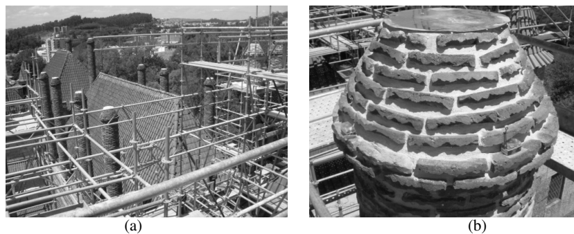
Figure 14: Chimneys at Paço dos Duques: (a) recent conservation works; (b) sensors location.
