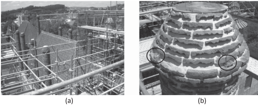
Figure 21 Chimneys at Paço dos Duques: (a) recent conservation works; (b) sensors location.
