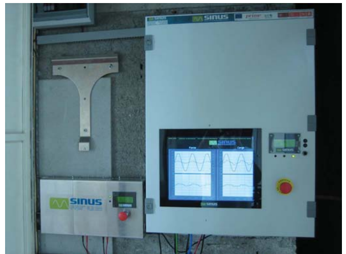
Fig. 7. MPPT and Shunt Active Filter installation
