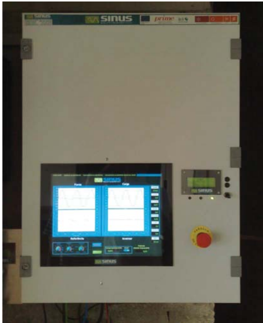
Fig. 4. Shunt Active Filter electric board installed in University of Minho
