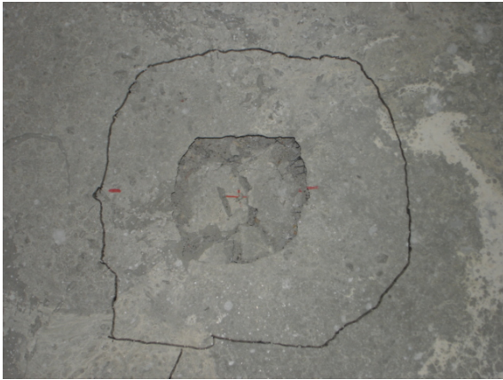
Figure 4.19: Punching critical contour and yield line due to negative moments (exterior contour)
