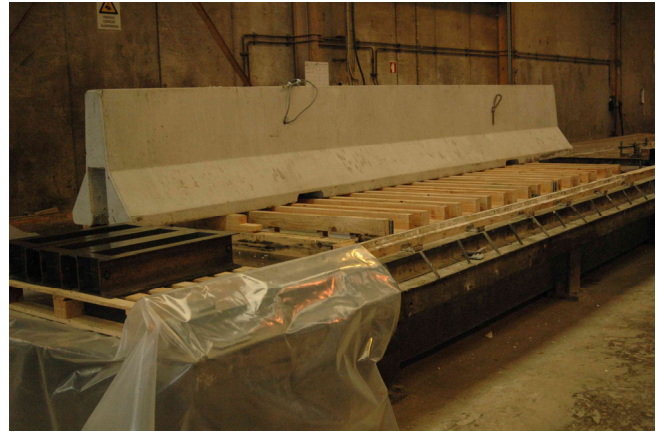
Figure 5.3: Heavy beam to assure stability of the lightweight elements during concrete casting
