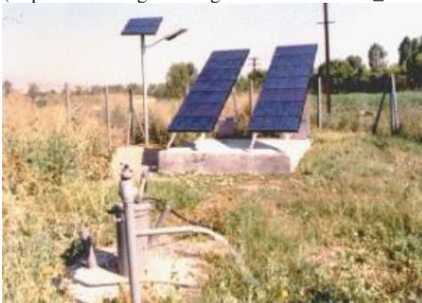
Figure 4.25. Photovoltaic Water Pumping Systems ( http://www.eie.gov.tr/english/solar/solarEIE_e.html )
