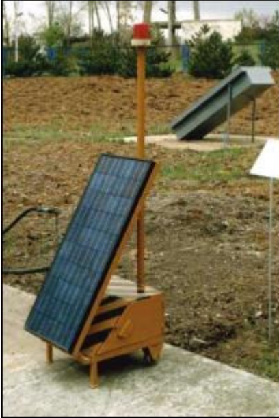
Figure 4.26. Photovoltaic Traffic Warning System ( http://www.eie.gov.tr/english/solar/solarEIE_e.html )
