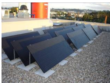
Figure 3.6. Hot water solar collectors (thermodynamic system).
