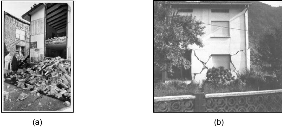
Figure 2.5 – Examples of damages caused by an earthquake in unreinforced masonry walls: (a) 1965 Seattle-Tacoma (Noson et al. , 1988) and (b) 1976 Friuli in Italy 4 .
