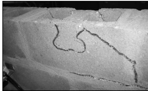
Figure 5.23 – Crushing of the concrete block under the load application point in specimen S-2C-SH.
