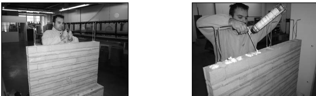
Figure 4.10 – Bending of the vertical bars and filling of the last course of wall with polyurethane foam.
