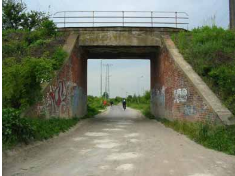
Fig. 2-14 Example of slab span with rectangular cross section and edge beams (photographed by the Author)
