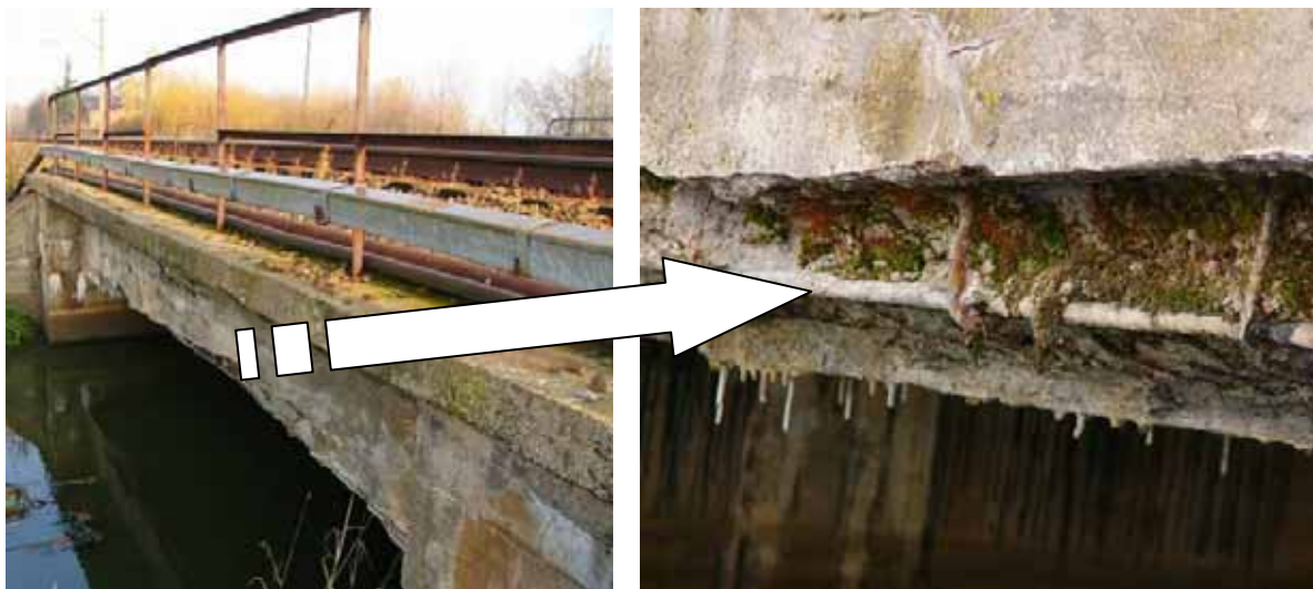
Fig. 3-12 Example of loss of concrete and protection (photograph courtesy of Jerzy Czastkiewicz, PKP)
