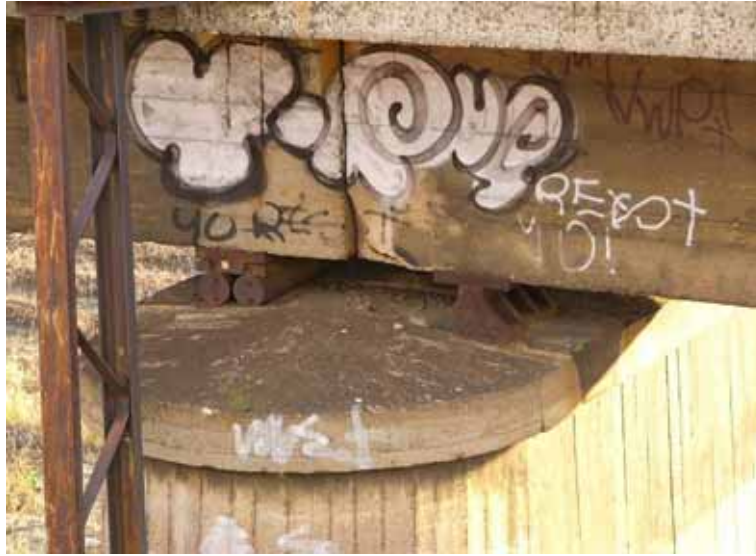
Fig. 3-4 Example of neutral inorganic contamination (photograph courtesy of Jerzy Czastkiewicz, PKP)
