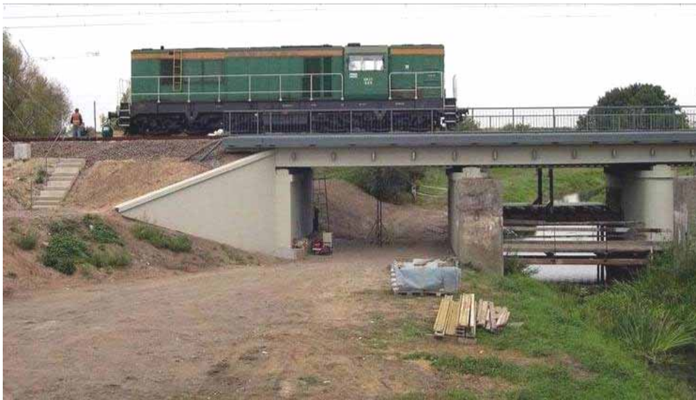
Fig. 4-26 Typical load test of railway RC bridge (photograph courtesy of prof. Jan Bień, WUT)
