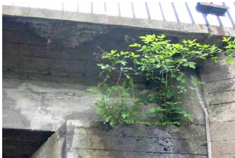
Fig. 5-20 Example of plants growing on concrete structure (photographed by Author)
