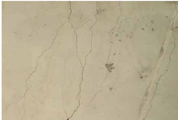
Fig. 5-10 Example fatigue of material effects – cracks in concrete (photographed by Author)
