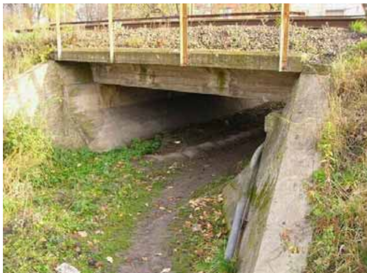
Fig. 2-13 Example of slab span with extended brackets (photograph courtesy of Jerzy Czastkiewicz, PKP)
