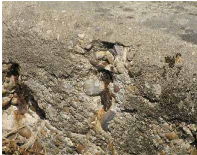
Fig. 3-13 Example of loss of concrete (photographed by the Author)
