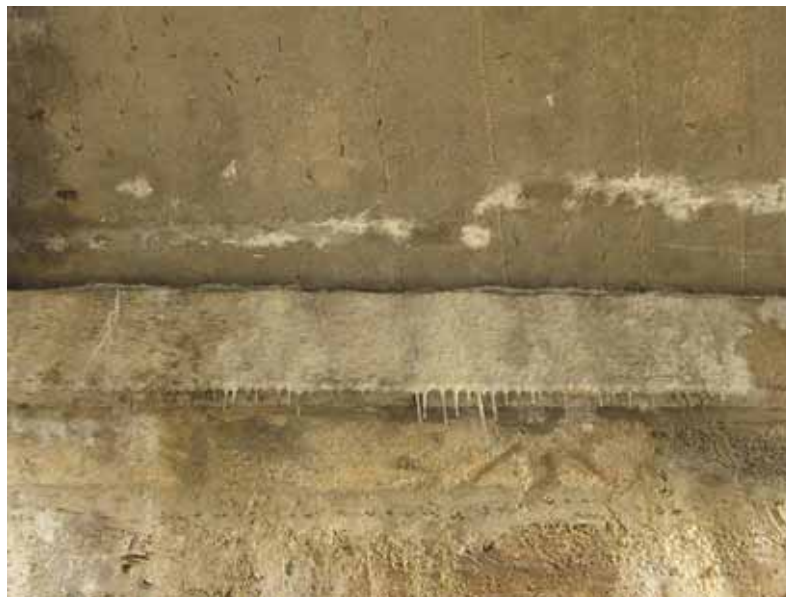
Fig. 5-7 Example of leaching effects – lime weeping (photographed by Author)
