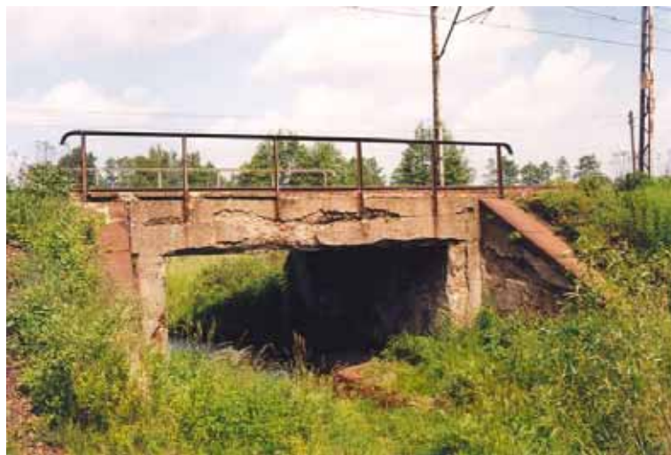
Fig. 5-3 Effects of carbonation of concrete (Stańczyk 2000)
