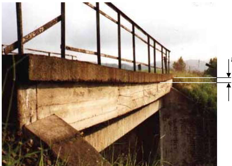
Fig. 3-5 Example of deformation: deflection (photograph courtesy of Zygmunt Kubiak, PKP)
