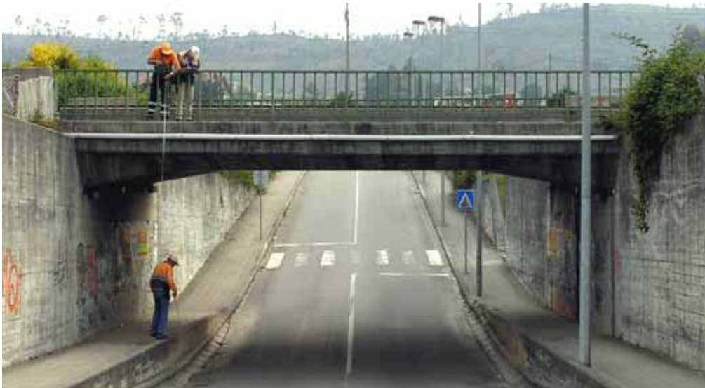
Fig. 4-25 Typical visual inspection performed by bridge inspectors from REFER (photographed by the Author)
