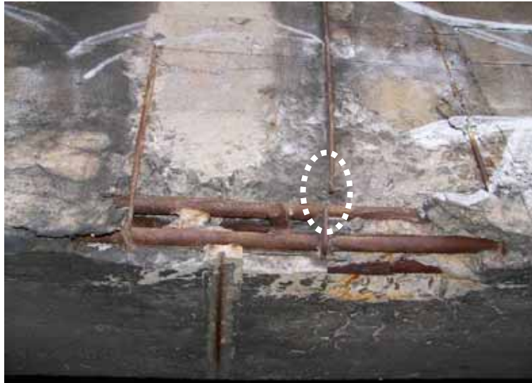
Fig. 3-9 Example of discontinuity: fracture of the stirrup (photograph courtesy of Jerzy Czastkiewicz, PKP)
