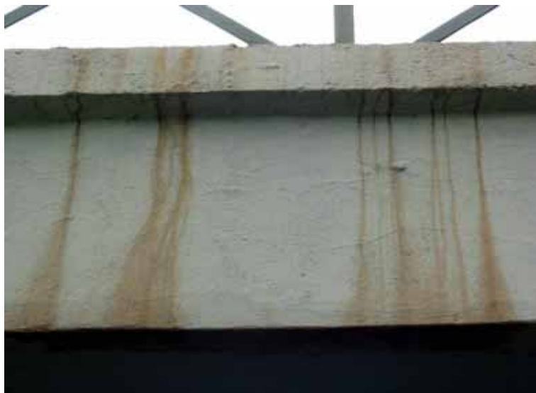
Fig. 3-3 Example of neutral contamination of concrete (photographed by the Author)
