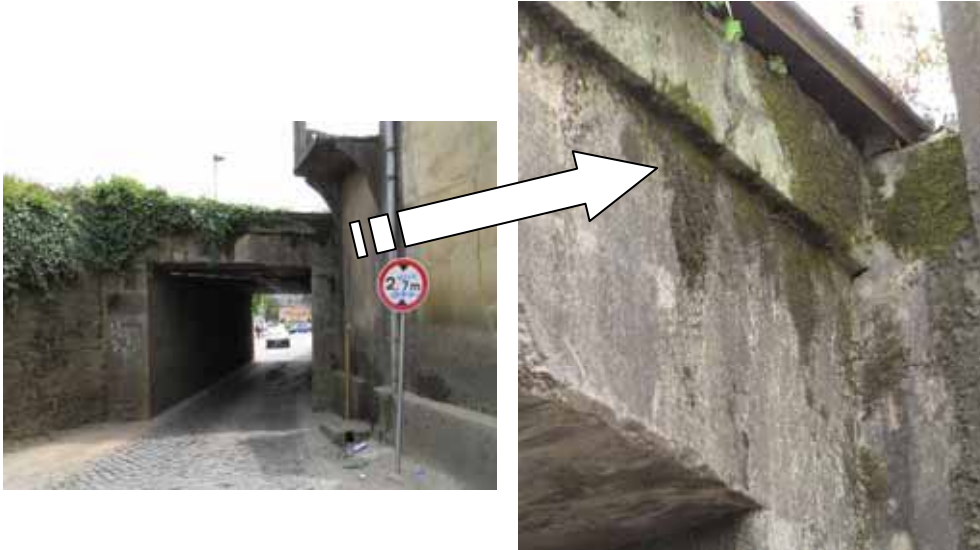
Fig. 5-19 Mosses on the concrete surface as an example of biological degradation mechanism effect (photographed by Author)
