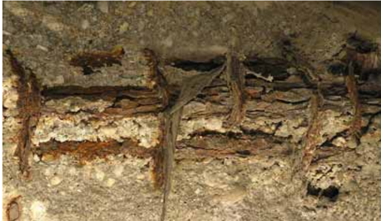
Fig. 5-5 Effects of corrosion at advanced stage with spalling of concrete (photographed by Author)
