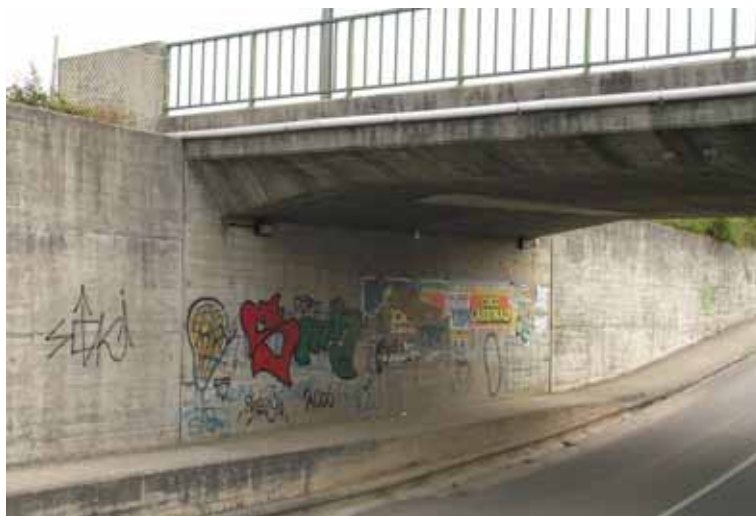
Fig. 5-17 Example of vandalism effects - graffiti (photographed by Author)
