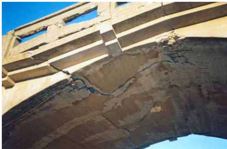
Fig. 5-15 Example of effects of overloading caused by earthquake (photograph courtesy of prof. Jan Bień, WUT)
