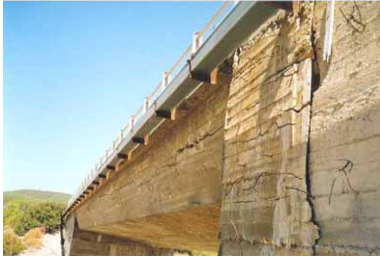
Fig. 5-16 Effects of shrinkage (photograph courtesy of prof. Jan Bień, WUT)
