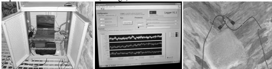
Figure 6: Dynamic monitoring system: datalogger, acquisition software and accelerometers
