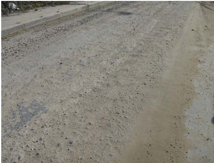
Figure 9 – Visible damage in the recycled material 8 days after opening to traffic
