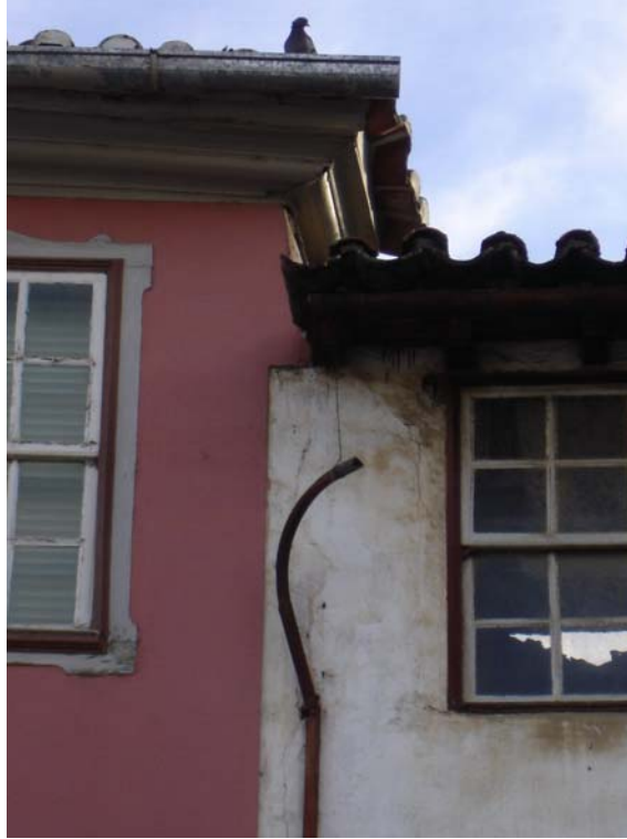
Figure 9 – Typical example of a defect in a downpipe.
