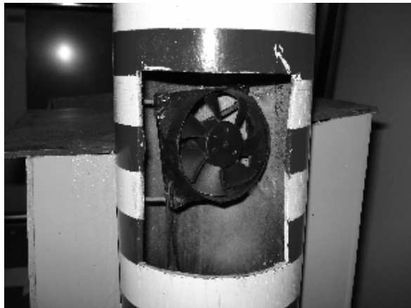
Figure 4. Fan inside the chimney
