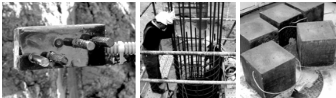
Figure 3. Images of the application corrosion sensors used and their installation.
