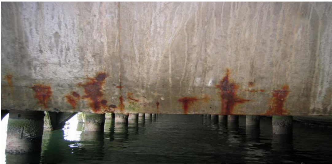
Figure 6.22 – Rust stains on beam 2.
