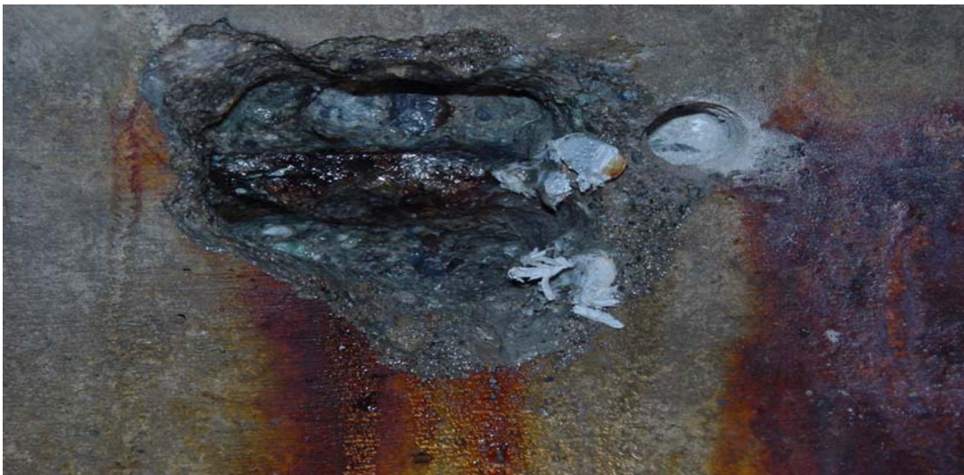
Figure 6.23 – Exposed reinforcement on beam 3.
