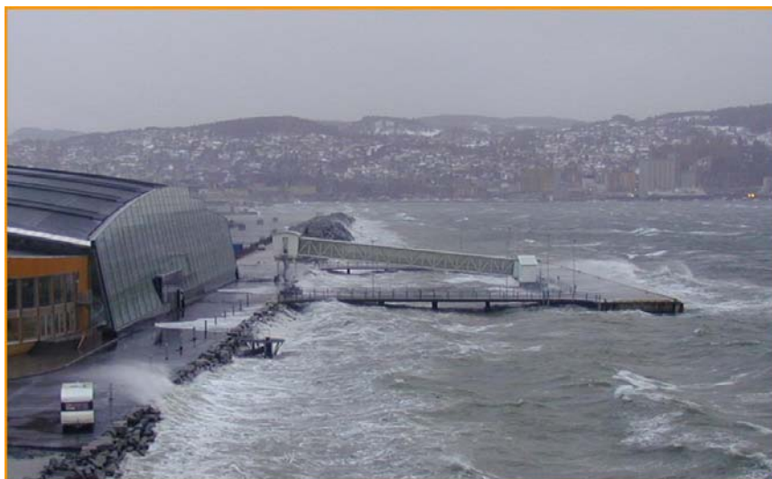
Figure 6.6 – A photograph of the concrete harbour structures investigated, suffering particularly severe weather.
