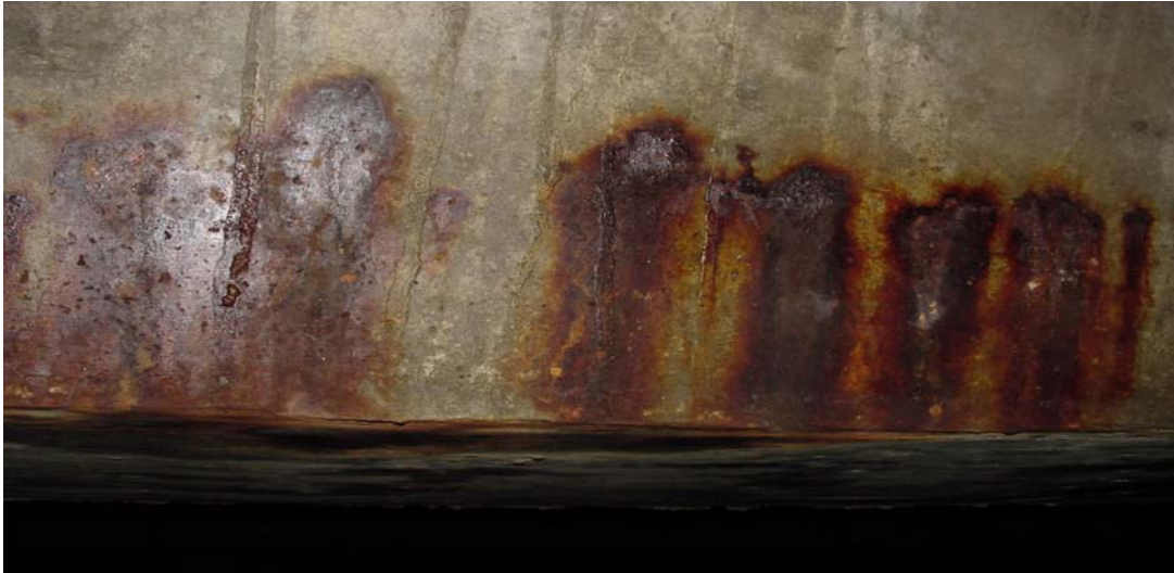
Figure 6.21 – Rust stains and corrosion cracking on beam 3.
