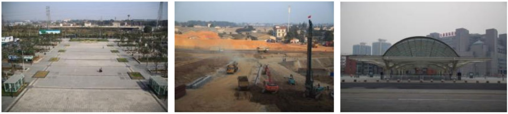
Figure 1. From left to right: Wuhan HSR Station entrance square; Construction site next to Guangzhou South Railway Station; Beijing South Railway Station entrance square. Source: author taken in 2012.
