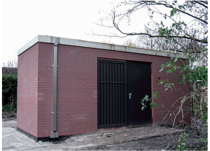
Image of an area point of presence, used for aggregating thousands of Internet connections whilst being protected with a simple lock
