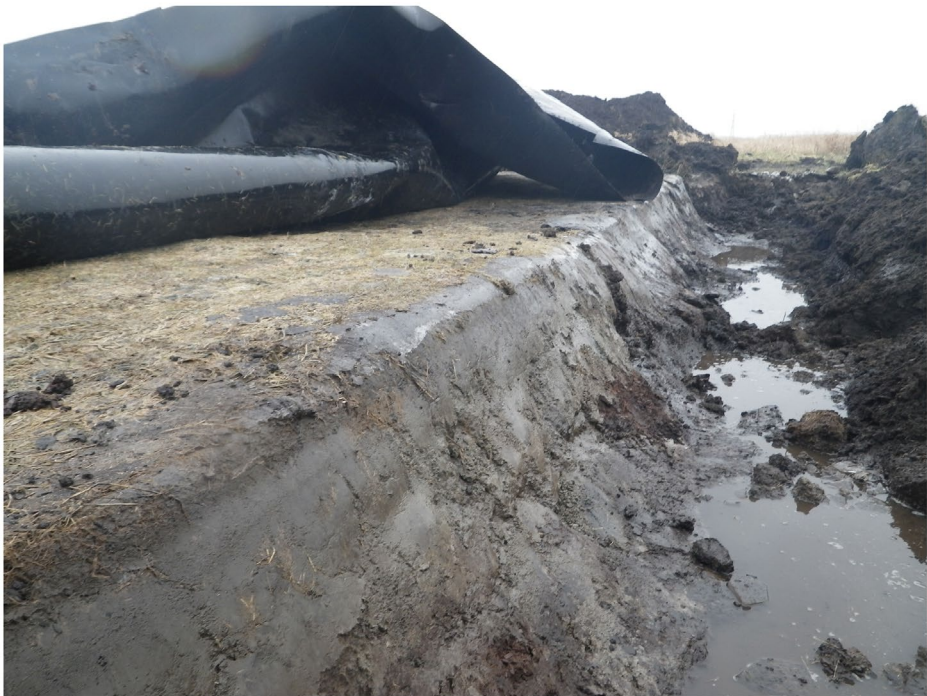
FIGURE 4 Compressed soil after removal of plastic cover and earthen load in February 2011.
